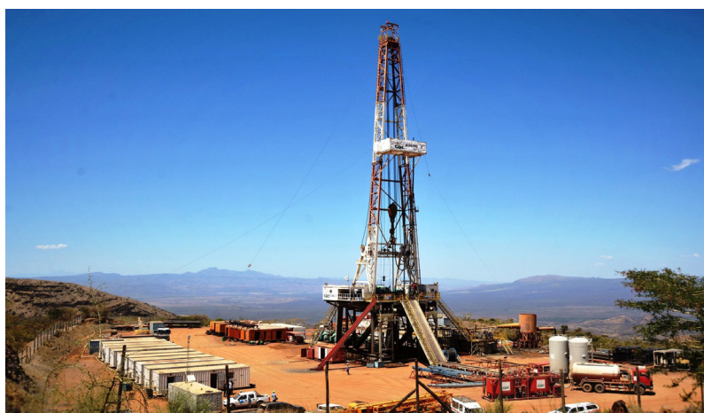
A Geothermal Development Company Rig in Silale Ward, Tiaty Sub County of Baringo County.
