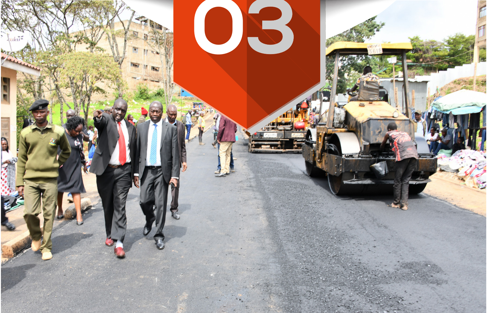
A County official updates Governor Benjamin Cheboi on the progress of paving one of the roads in Kabarnet town during a project inspection tour within the urban area
