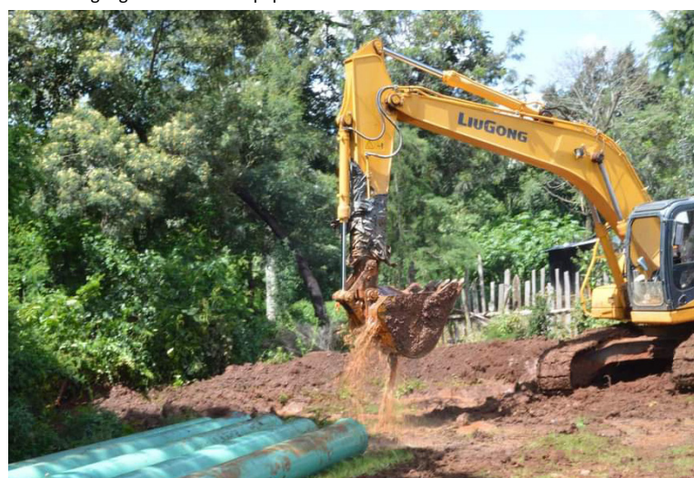
An excavator at work during the laying of pipes to supply water from Chemosusu Dam in Eldama Ravine
