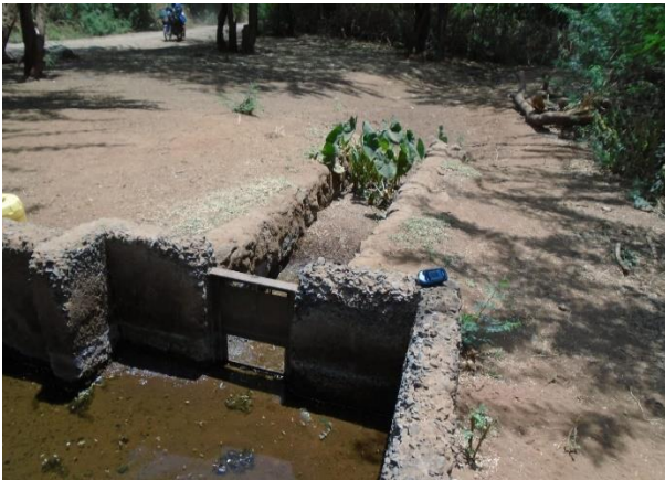
A dry intake in Kapkuikui
